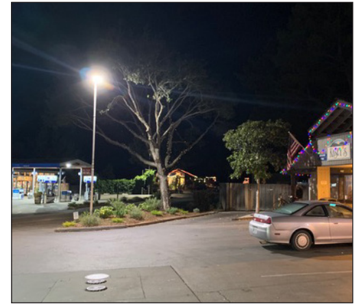
Sodium light on parking lot pole cast light over large area.
