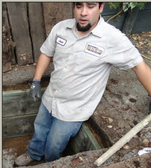
Local tank reconstruction, with a worker from Peninsula Septic Tank Service Inc. Photo by Mibs McCarthy
