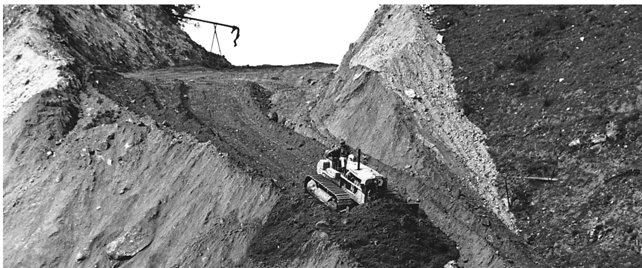
A caterpillar tractor breaks through the last ridge over Laureles Grade as the road is built in the 1940s. — photo from the collection of Tom Augustitus
